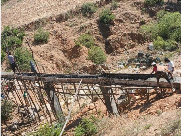
Construction work has already begun on a canal that will later carry the water from the dam to the fields. The aqueduct crosses a ditch.
